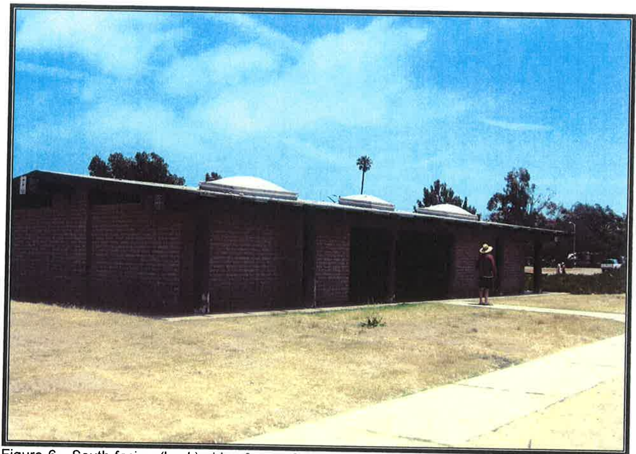
Figure 6. South-facing (back) side of one of two restrooms that would be replaced by a single, smaller combination building (102 m 2 [1,100 ft 2 ]) in the Day Use Area at Carpinteria State Beach.
